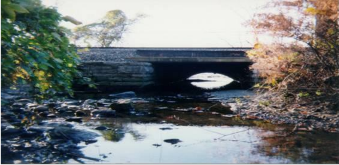
Photo 5 – View looking west at low tide at mouth of Wickers Creek, Showing outlet under the Amtrak/Metro North Railroad
